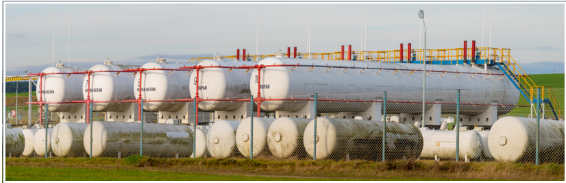
Fig. 148: Liquid gas tanks
