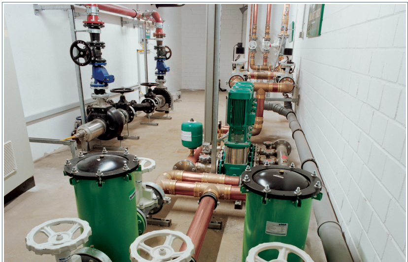
Fig. 100: Viega piping system Sanpress XL in a water treatment plant
