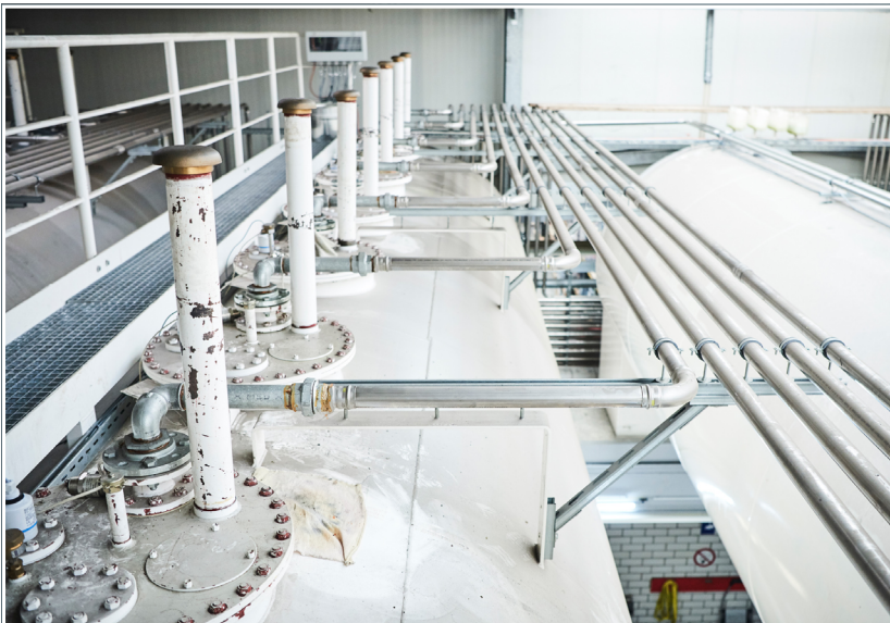
Fig. 174: Cooling lubricant tanks filled and emptied using Viega Sanpress Inox G
