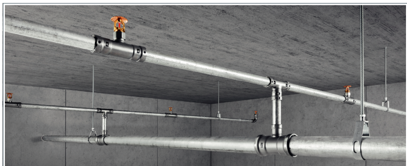
Fig. 112: Sprinkler unit with Viega Megapress and galvanised steel pipe
