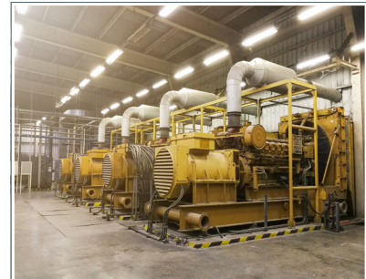
Fig. 170: Diesel-operated emergency generator
