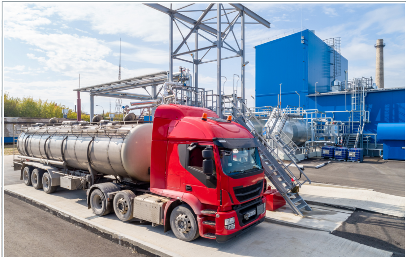
Fig. 172: Filling plant for diesel fuel
