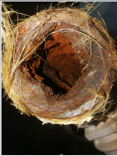
Fig. 74: Galvanised steel pipe with clearly visible corrosion
