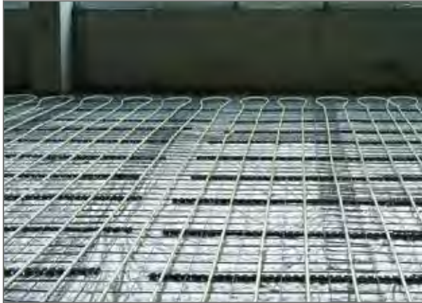
Fig. 227: Fonterra Industry, installation example
