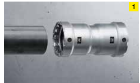
The steel pipe is cut to length and cleaned. Then the insertion depth is measured and marked, then the Megapress connector is put on the pipe up to the mark.
